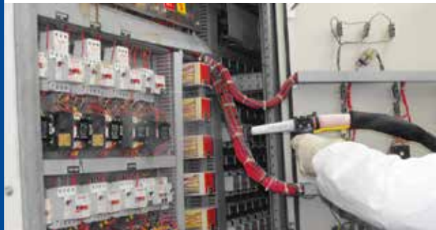
Electrical cabinet cleaning
