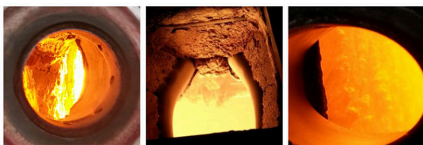
Superheater Pendant - Before Cleaning
